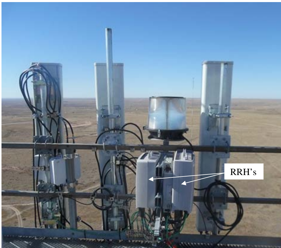
Figure 3: RRH's Positioned behind the Antennas
