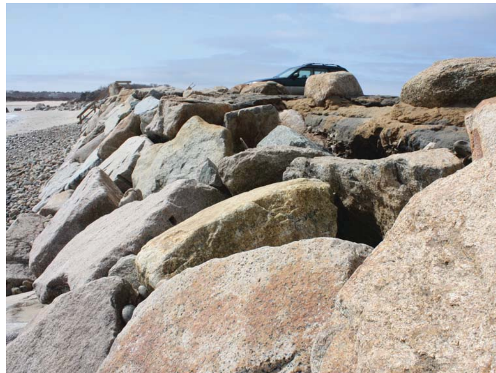
5 – Revetment settlement following severe storm event
