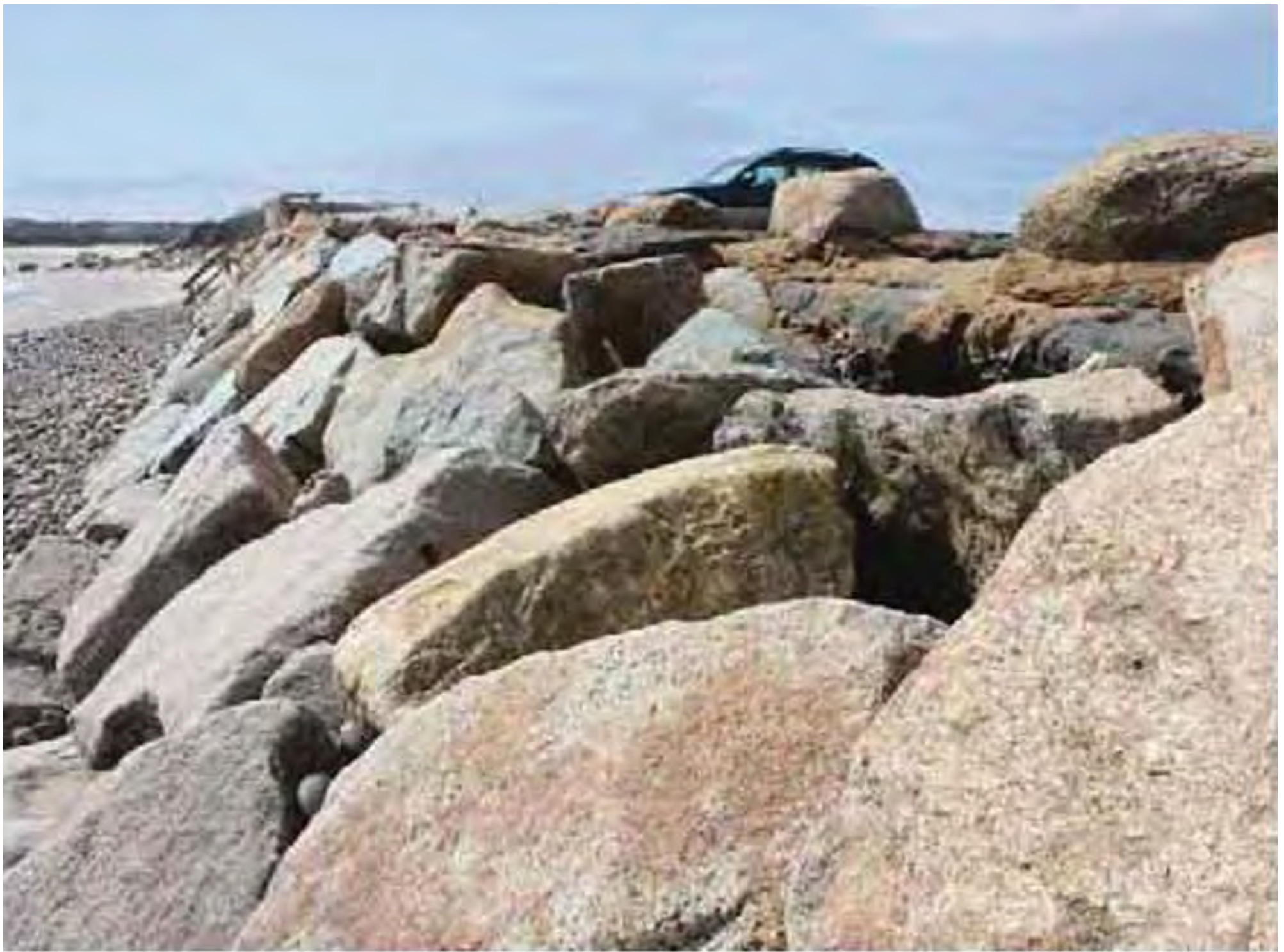
5 – Revetment settlement following severe storm event
