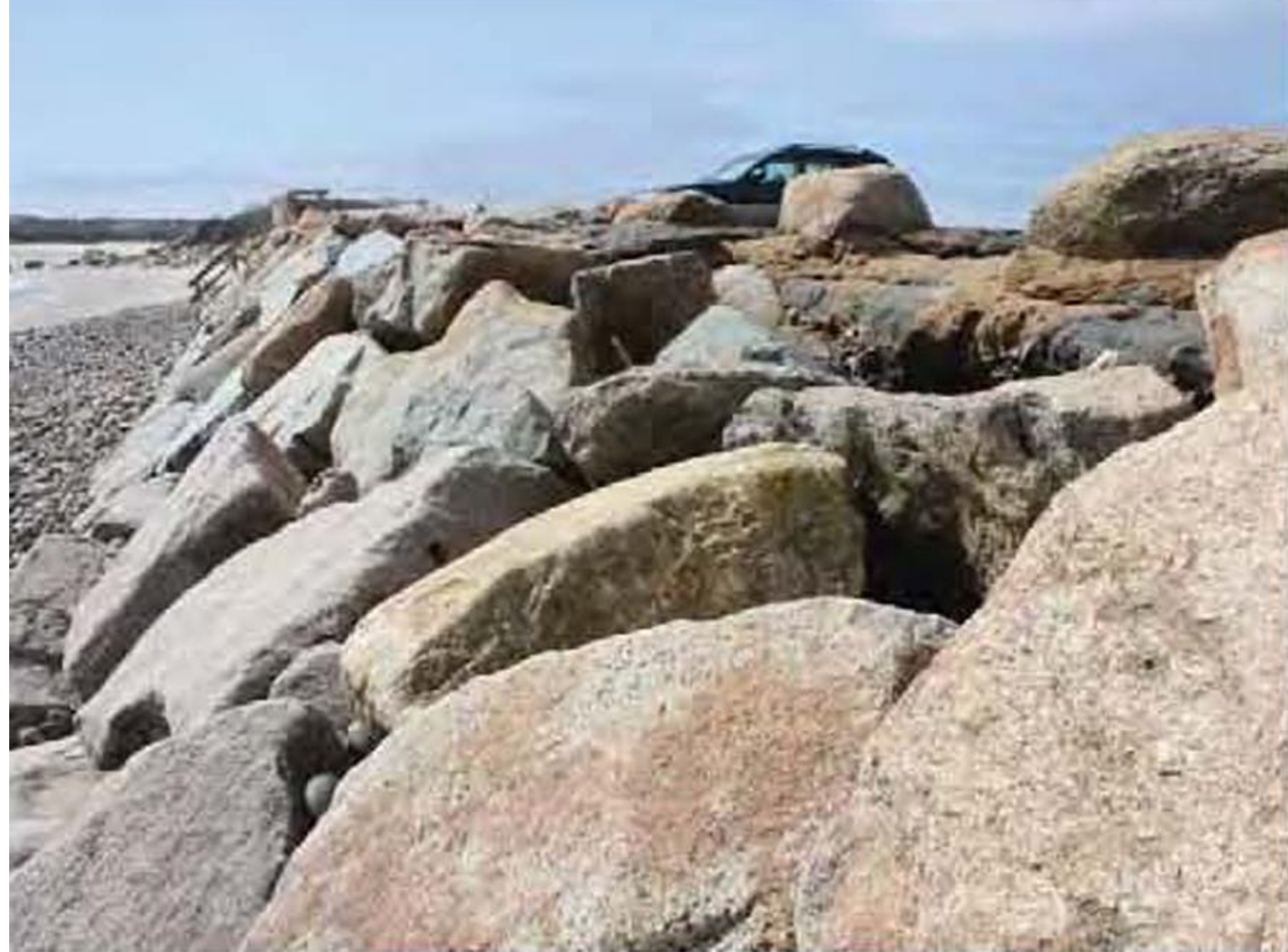
5 – Revetment settlement following severe storm event
