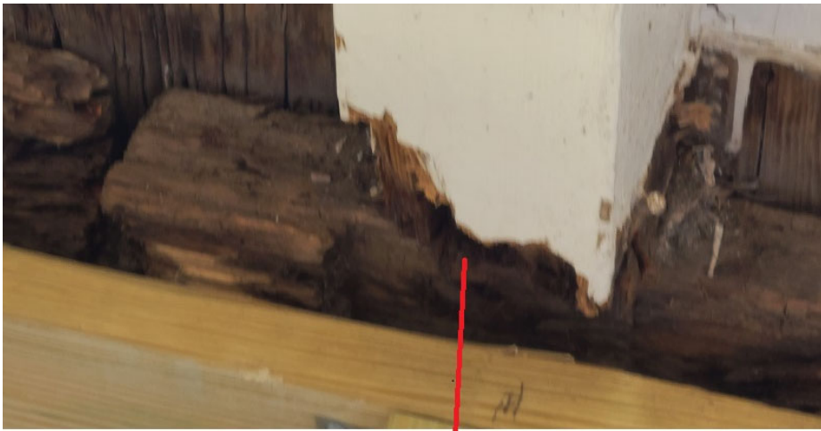
Example of one of the posts that has rotted.
