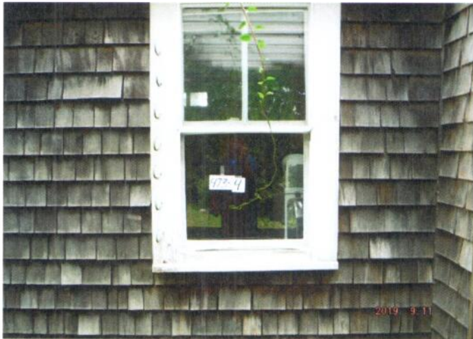
Sample 473-4 Middle back window Caulking
