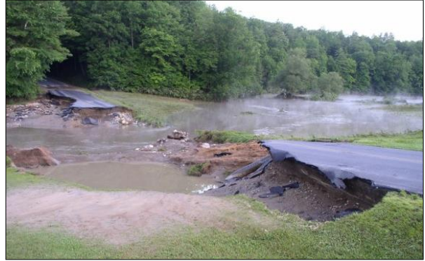
Damage from Hadlock Pond Dam failure, Fort Ann, NY
