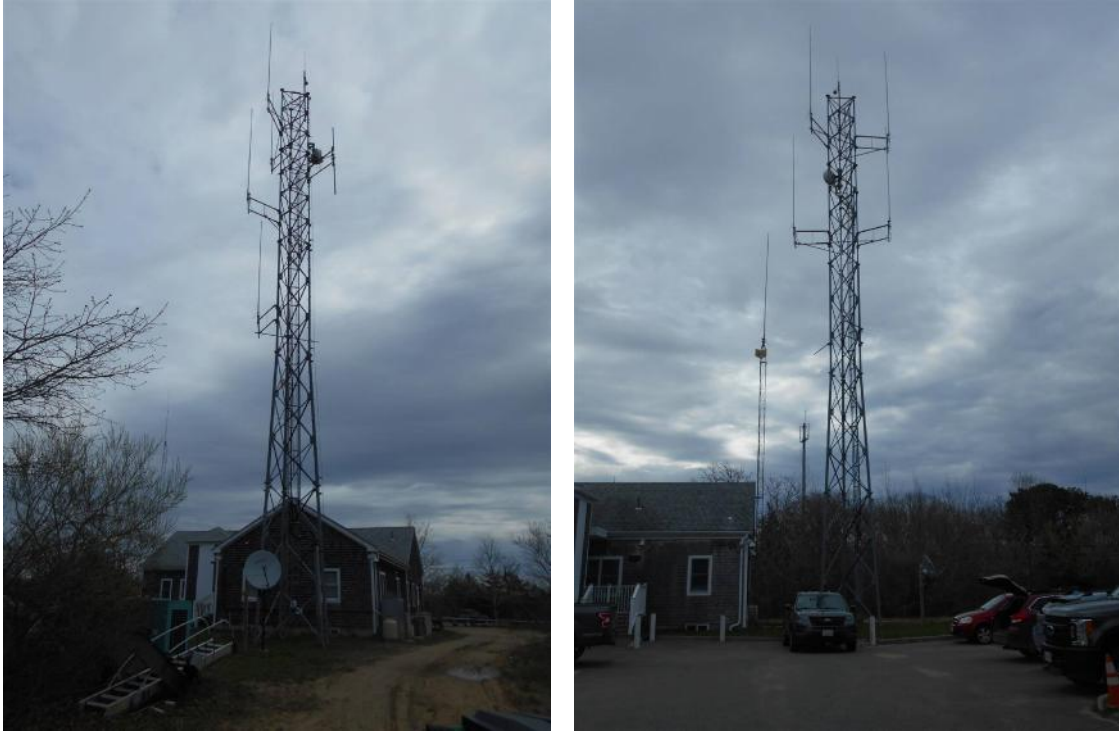
Overview photos of 95' self-supporting tower
