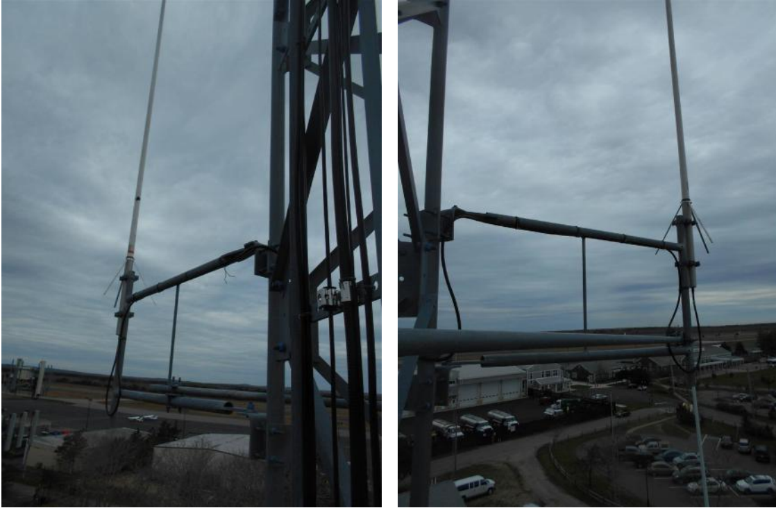
Additional equipment and mount photos
