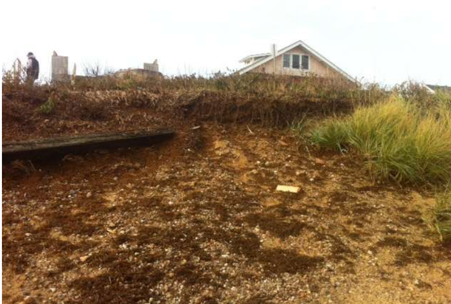
NORTH BLUFF BANK DAMAGE DUE TO HURRICANE SANDY 2012
