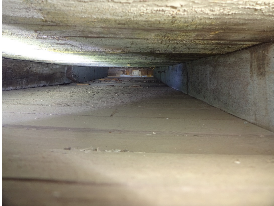
Figure 3: Sagging Rafters Below East Dormer
