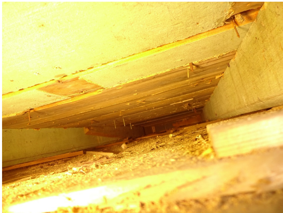
Figure 5: Floor Shimming @ NE Corner of Main Structure
