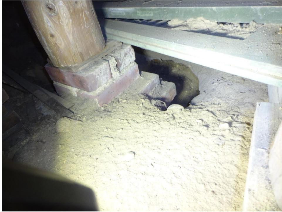
Figure 10: Undermined Brick Pier
