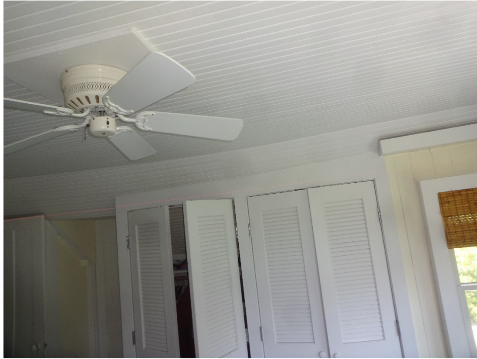
Figure 13: Second-Floor Roof Sagging along the Master Bedroom Closet Wall
