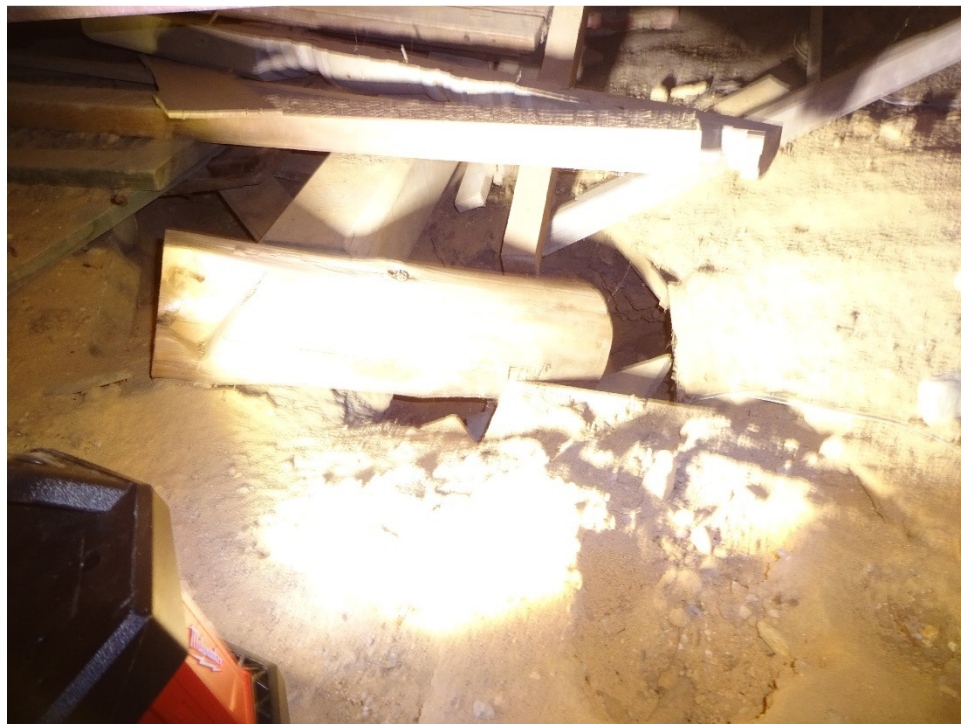
Figure 11: Dislodged Support Column
