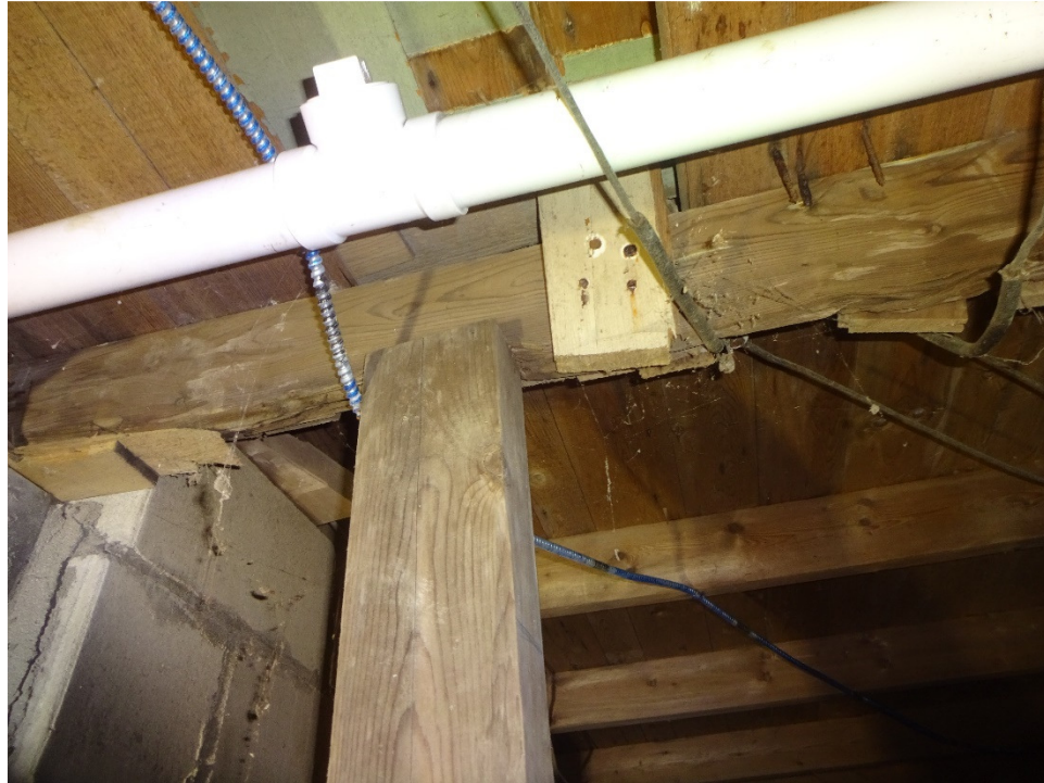
Figure 6: Deteriorated Floor Framing and Temporary Support Post
