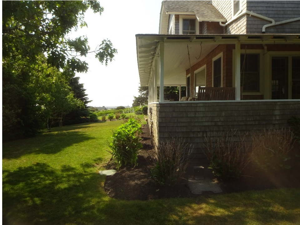
Figure 15: Bowed Framing Along East Side of Existing Structure
