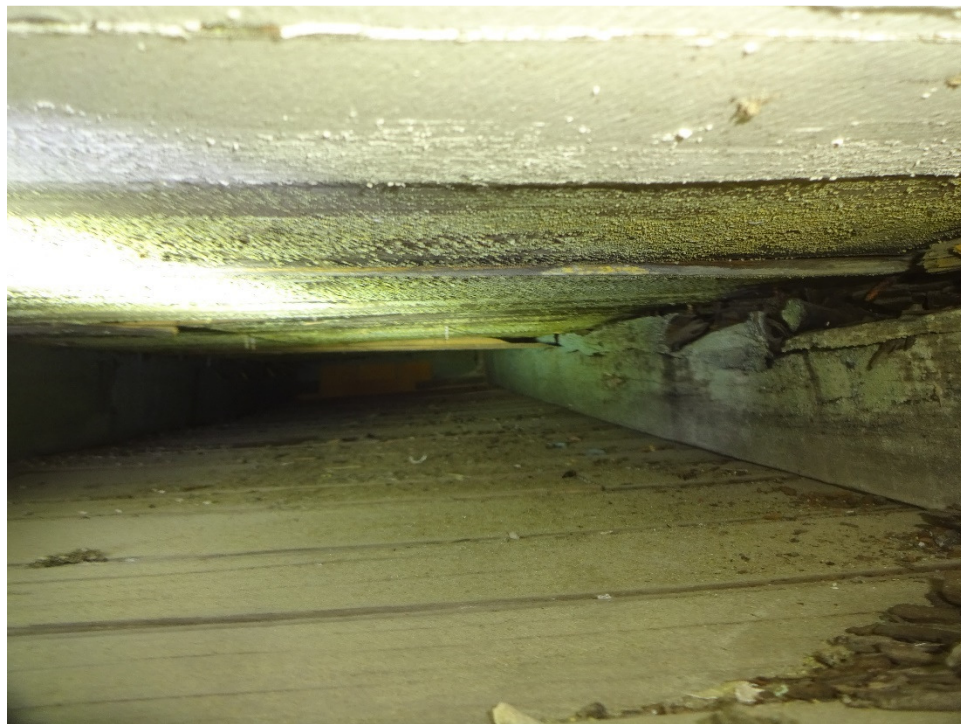
Figure 2: Damaged Rafter Adjacent to South Chimney
