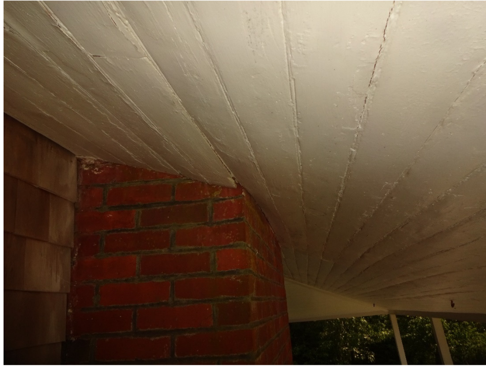
Figure 1: Porch Ceiling Sagging Around South Chimney
