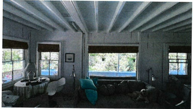
Load bearing wall showing 4x4 posts spaced far apart with minimum exterior shear capacity. Deflecting rim joist/header is also evident from this photo.
