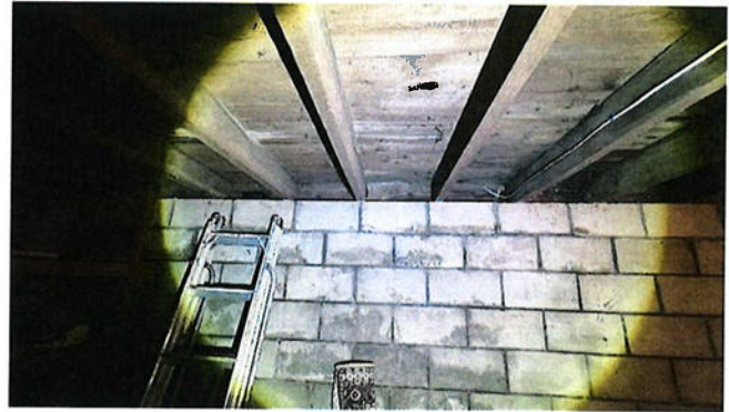
True 2x4 joists indicate construction of entire 1 st level floor was after 1900
