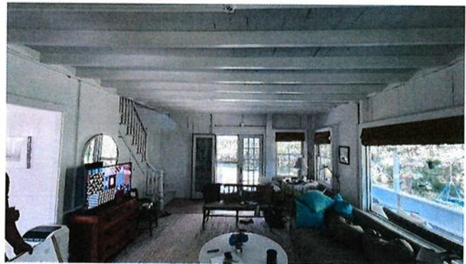
3x6 joists showing significant deflection and over stressing
