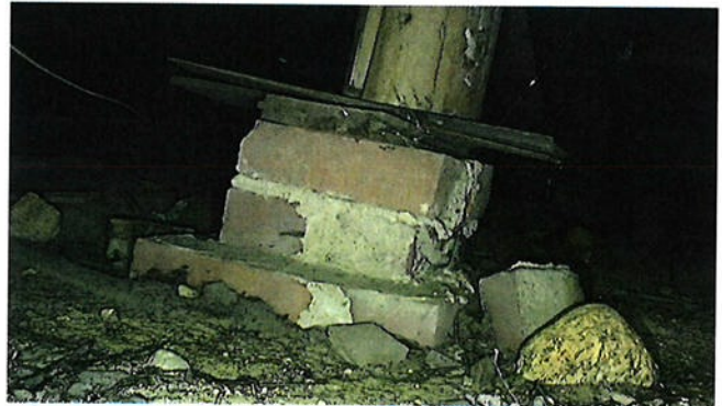
Inadequately supported timber pier with brick footing/wooden shims
