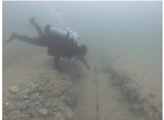
Fig. 2. Cable trench in cemented sediment at dive site 2 in June 2005, approximately 12 months after cable laying. The linear feature in the trench is a measuring tape (Photo: CEE Consulting).
