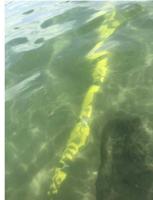
An exposed section of the cable is seen here about 3' below the water at low tide.
