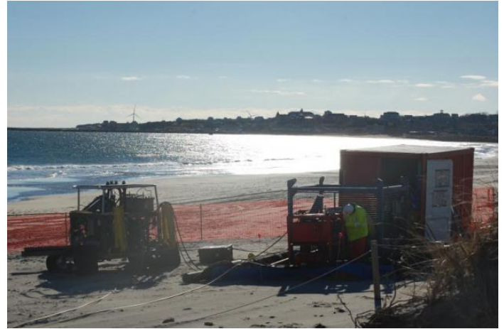
Crews from National Grid and Ørsted U.S. Offshore Wind are surveying the cables at Fred Benson Town Beach to study how best to reach a long-term plan to bury the cables to their appropriate length. Photo by Lars Trodson
