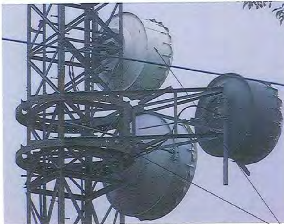
THE (3) DISHES AND MOUNTS FROM 55' TO 65' ARE TO REMAIN ACTIVE DURING CONSTRUCTION. THE ANGLE-X FROM 45'-4" TO 65'-2" IS TO BE INSTALLED LAST SO THESE DISHES CAN REMAIN ACTIVE. ONCE ALL OF THE REINFORCEMENTS AND TOWER EXTENSION HAVE BEEN INSTALLED RE-LOCATE THESE (3) DISHES AND MOUNTS TO THE TOWER EXTENSION. AFTER THESE DISHES AND MOUNTS HAVE BEEN RE-LOCATED TO THE TOWER EXTENSION THE ANGLE-X FROM 45'-4" TO 65'-2" IS TO BE INSTALLED.
