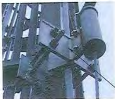
EXISTING SAFETY CLIMB TOP TERMINATION AT 33' TO BE REMOVED PRIOR TO ANGLE-X INSTALLATION.
