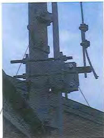
EXISTING SAFETY CLIMB BASE TERMINATION TO BE REMOVED PRIOR TO ANGLE-X INSTALLATION.
