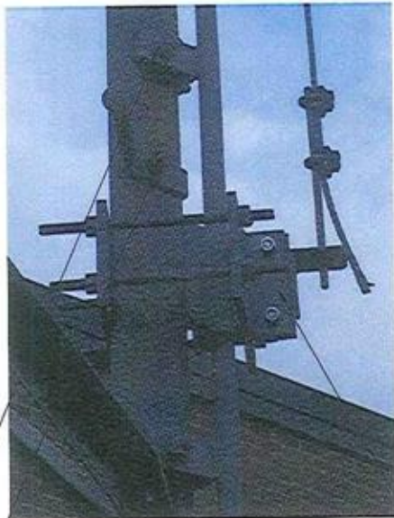
EXISTING SAFETY CLIMB BASE TERMINATION TO BE REMOVED PRIOR TO ANGLE-X INSTALLATION.
