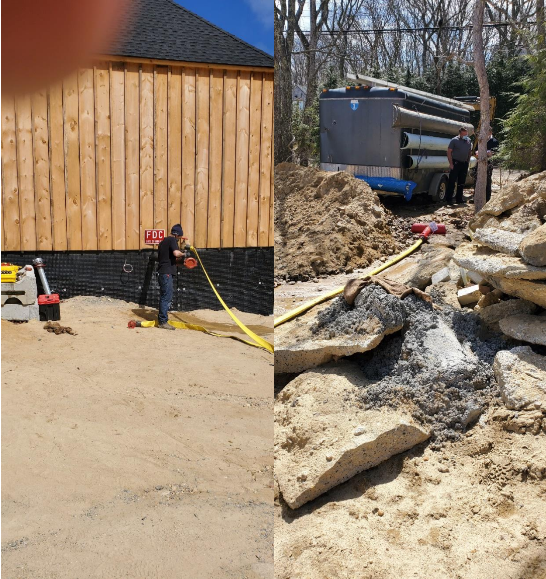
Test manifold set up at the FDC location.
