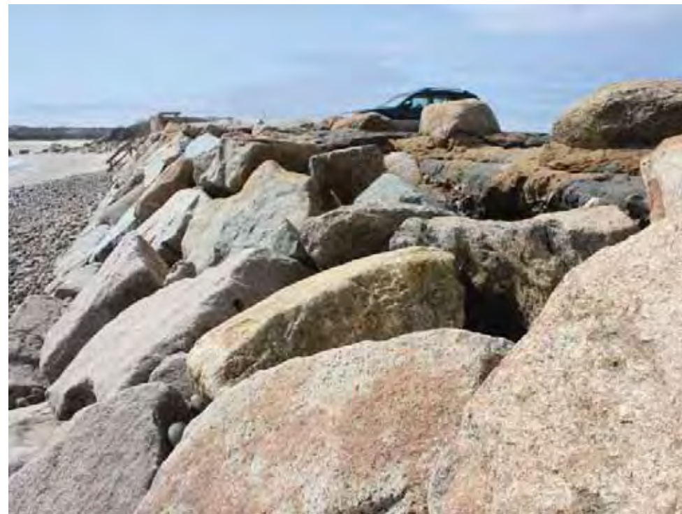
5 – Revetment settlement following severe storm event
