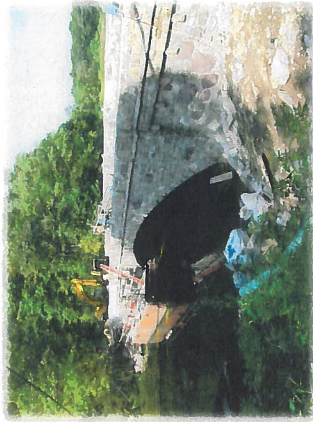
Between Dover and Needham, the Willow Street Bridge has been replaced using a precast arch, faced with stones from the original bridge to maintain its historic character
